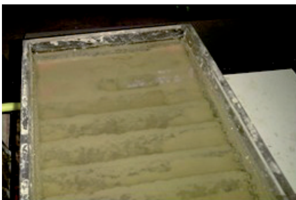
Fig. 7. Photo of anammox in the secondary clarifier.
