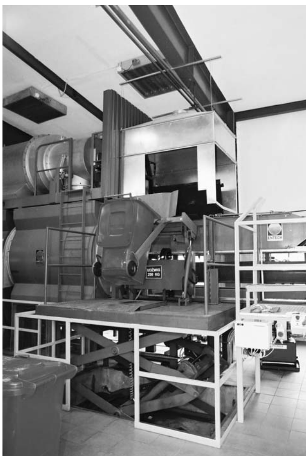
Fig. 1. Waste handling system at the Oncological Hospital in Bydgoszcz.
