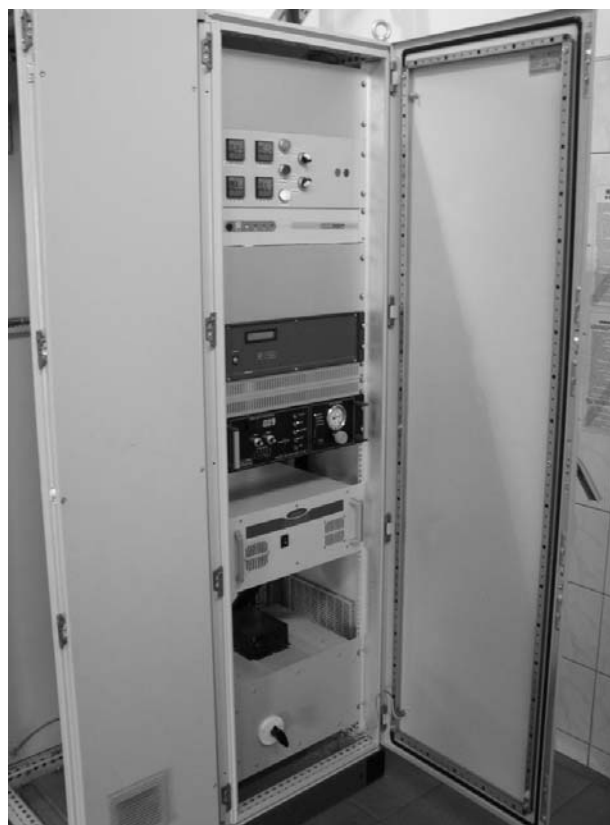
Fig. 4. Gas sampling system (measurements of flue gas fluxes and dustiness).
