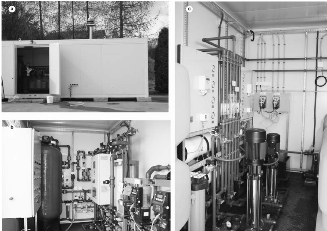
Fig. 5. Pilot geothermal water desalination facility at the PAS MEERI Laboratory: a) container housing the pilot facility; b) water pre-treatment stage: control panel and iron removal stage (left), ultrafiltration module and chemical dosage equipment for ultrafiltration (right); c) two-stage reverse osmosis arrangement with high-pressure pumps (centre).
