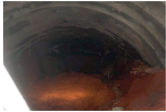
Fig. 5. Collapse situation of tunnel face YK169+212.
