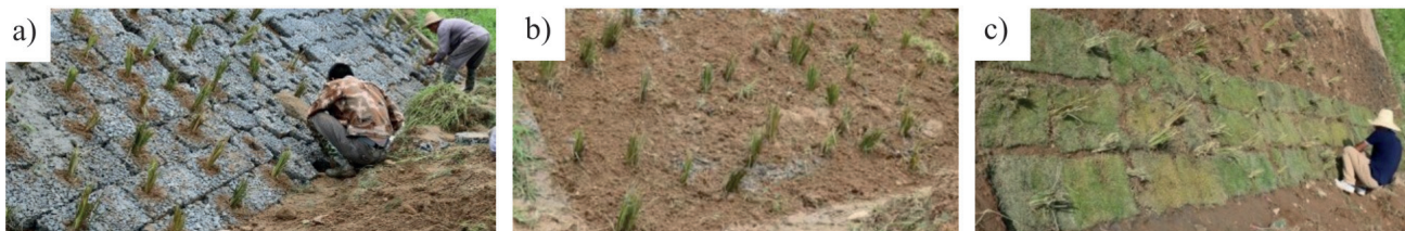
Fig. 11. Process of construction (a) Set up of prefabricated grass-planting concrete; b) Covering soil; c) Covering Bermudagrass turf and planting Vetiveria ).
