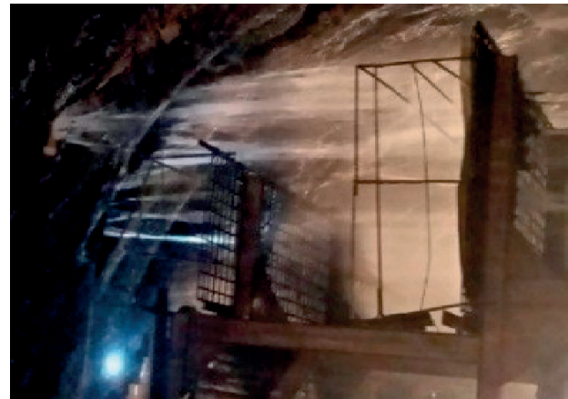
Fig. 4. Water inrush situation of the river-crossing section in the Yuelongmen Tunnel [31].
