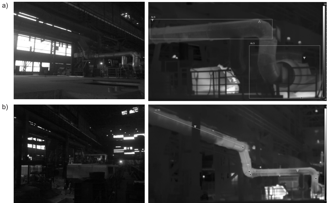
Fig. 7. Thermo-grams of pipelines for cooling and ventilation systems.
